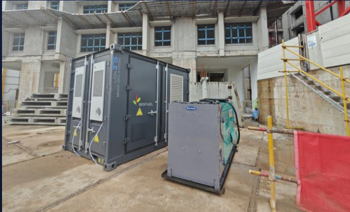
Diesel generator and energy storage complementary
