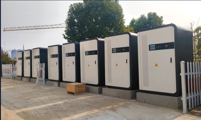
Full power operation at 1000V DC
