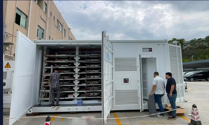
Second-life utilization of power batteries
