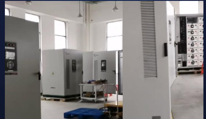
Off-grid switching with 4 STS modules in parallel
